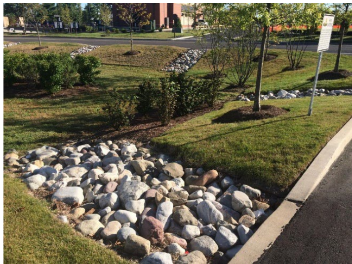
Figure 9. Rain Garden Features - Wegman's Parking Lot, Montgomeryville PA (PEC)
