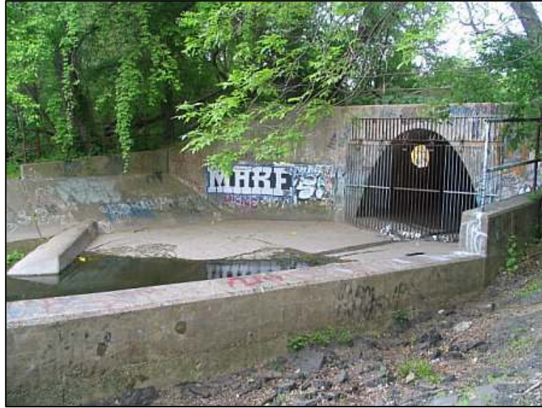
Combined Sewer Overflow in Tookany-Tacony/Frankford Watershed, Philadelphia
